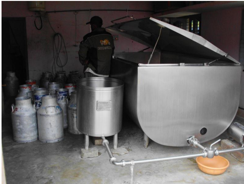
FIGURE 1. Bulk Milk Chiller
